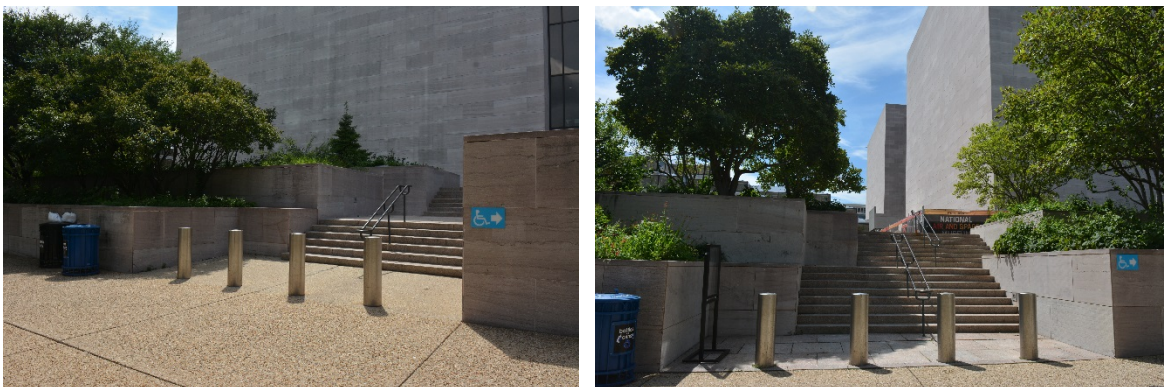
Figure 21: Retaining walls and stairs create and connect tiered terraces throughout the site, 2016 (EHT Tracerics).
