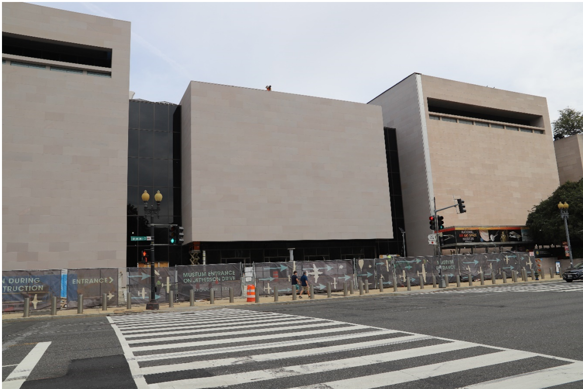
Figure 11: South elevation, cantilevered, masonry-clad block at glass bay, facing north. New granite cladding visible at center and left, October 2021 (Smithsonian).
