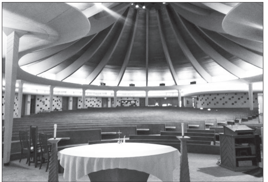
Two years ago, moldy carpet and rotted wood were removed from the sanctuary, spacious enough to seat 700. Since then, the pews that had been covered in carpet as part of the architectural design have been removed.
