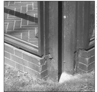
Broken brick and other deterioration
