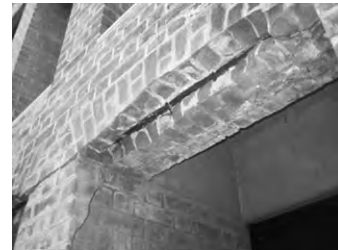
Detail: Steel and Brick Spalling (photo: Kees Spanjers)
